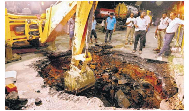
Water leakage from pipeline may have led to cave-in on Greems Road | MARTIN LOUIS
