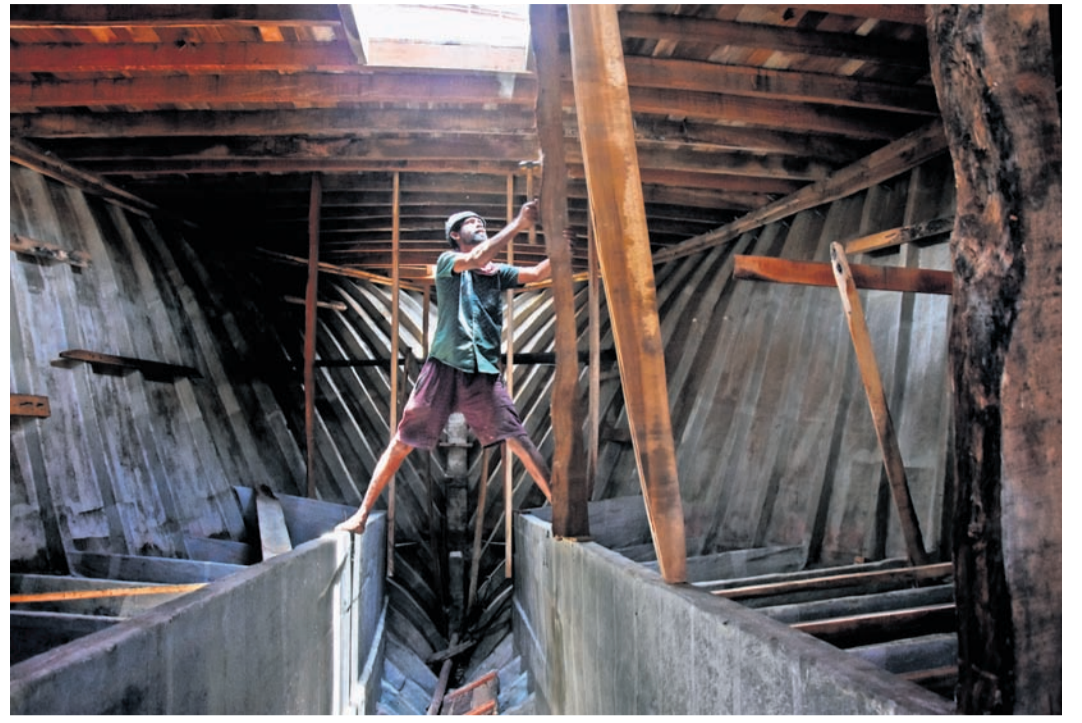
SEAWORTHY A carpenter works away on a mechanised fishing trawler at Kasimedu harbour on Wednesday during the annual fishing ban period | ASHWIN PRASATH
