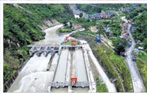
A hydropower plant and one under construction plant, all nested inside
