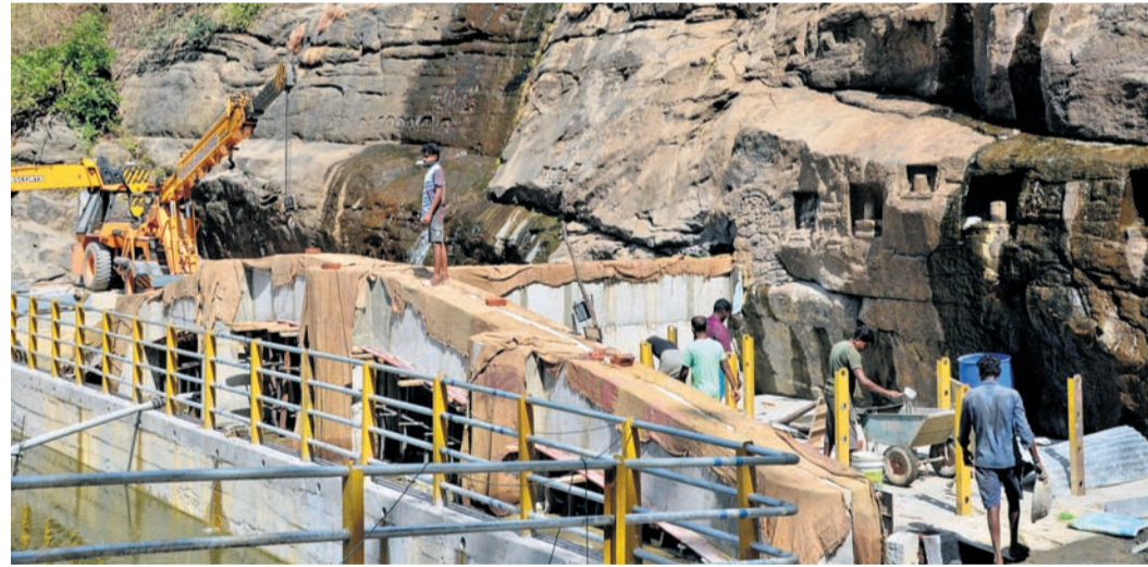
Renovation works in full swing at the Courtallam Main Falls in Tenkasi on Tuesday, ahead of the tourist season | V KARTHIK ALAGU
